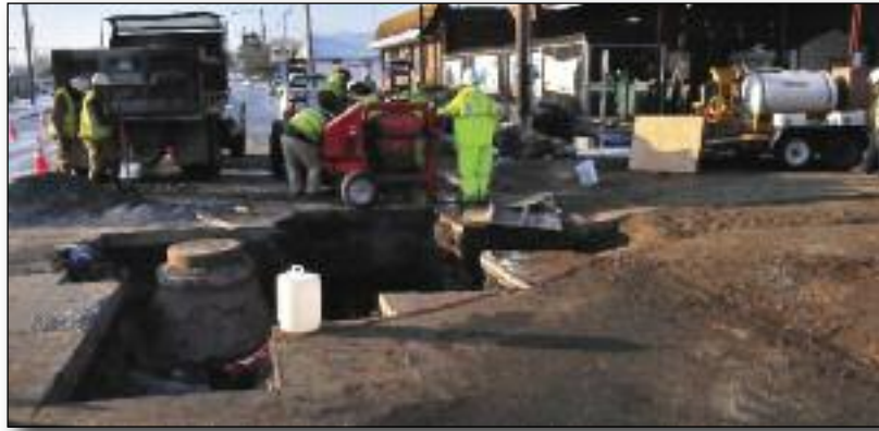
FPU water and gas crews work together to make repairs to the 12-inch wastewater line that runs across South Main Avenue. Their teamwork sped the efforts to make repairs.
